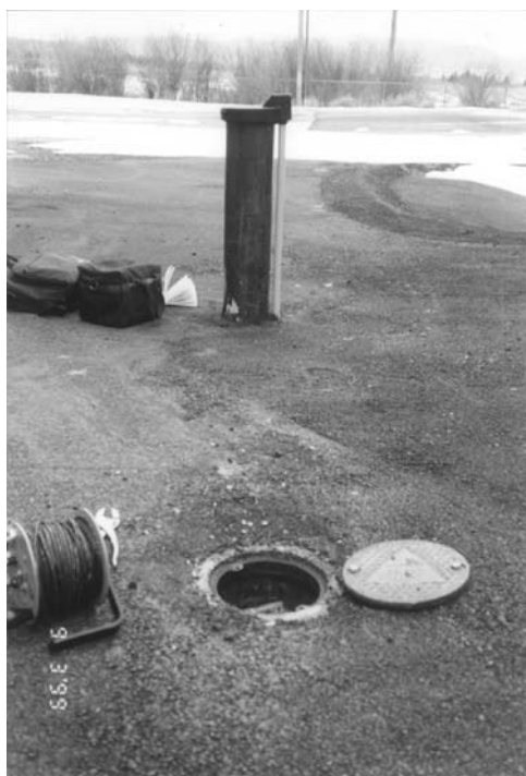
Figure 26.2 Pumping well and monitoring well with flush mount security plate.
