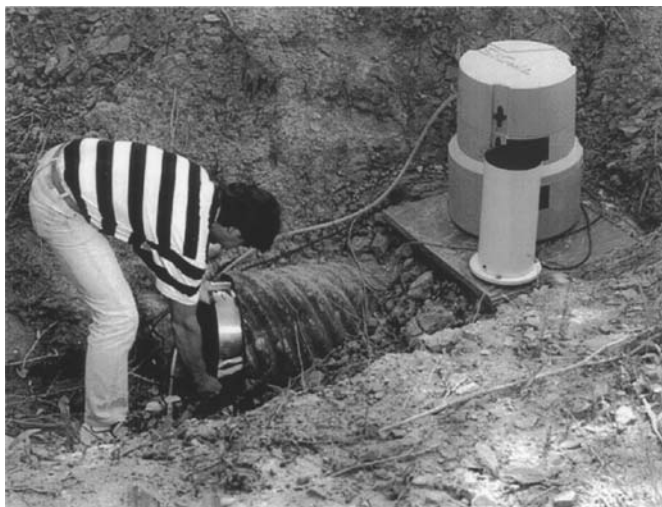
Figure 35.4 Storm water setup.
