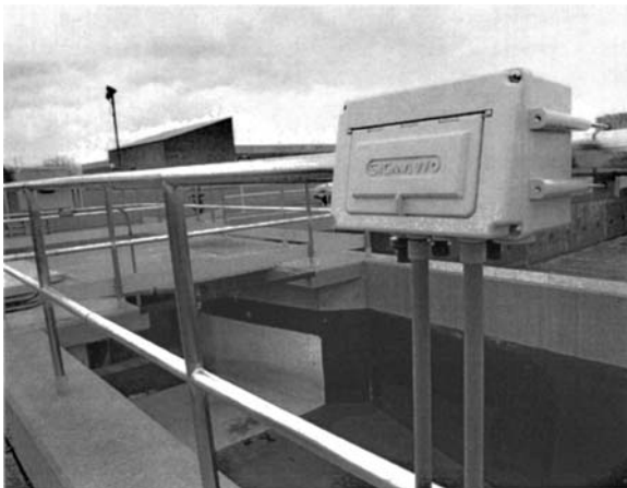
Figure 43.8 Influent flow monitor.
