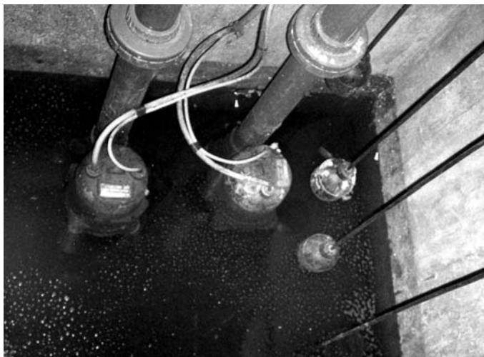
Figure 36.15 Float level controls for seal water sump, Massena Wastewater Treatment Plant, Massena, NY.
