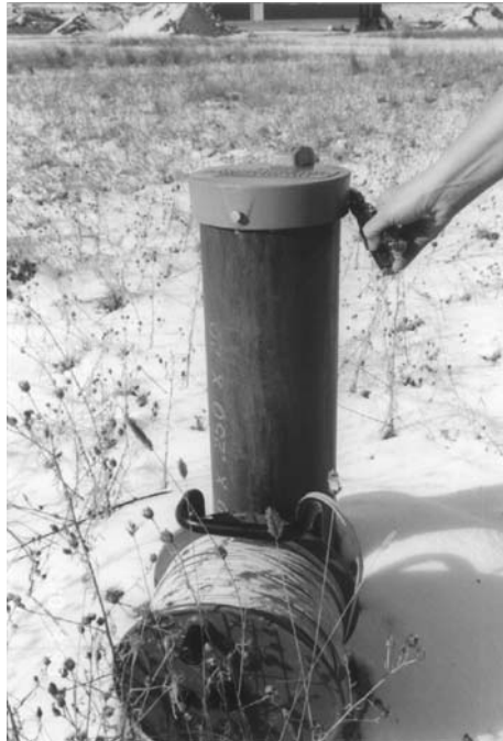
Figure 26.3 Domestic well cap secured with three bolts.
